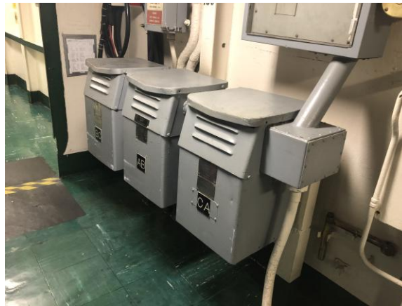
Figure 2: Transformer bank onboard USS Midway (CV-41)
